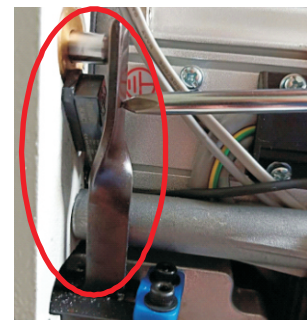
Fig. (12) After the Sensor Installation
